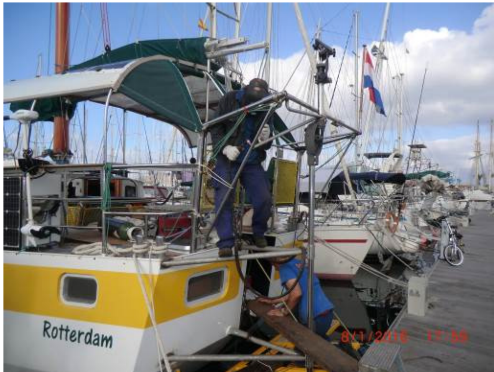
The welder and his helper busy making the brackets that support the Hydrovane. A courageous man, balancing above the water while he could not swim!
