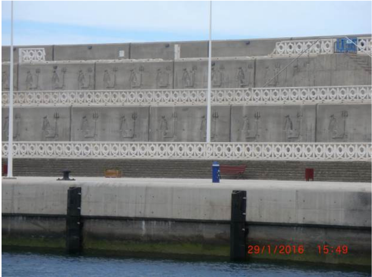
Water damage on the pier wall in Puerto de Garachico.
